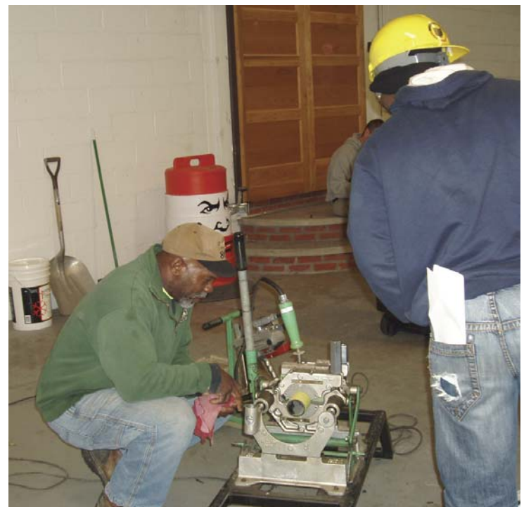
Eduardo K. Qadir, aka "Q," watching the iron heat the plastic pipe for a butt connection
