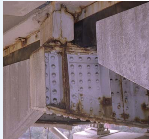
The rusting Innerbelt Bridge
