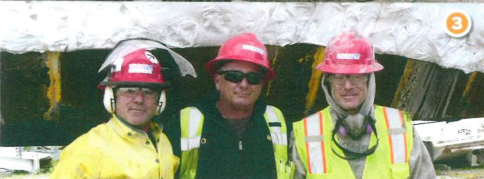
DUGWAY SEWER SALINI IMPREGGIO HEALY JV 1. Dan Steltenkamp, Rob Still, Neil McFadden and Reggie Palmer 2. Mike Wiemer, Adam Dailey and Lee Roberts 3. Giuliano Maddamma, Emiddio Colombo and Dave Foster 4. Marko Olivo 5. William McFadden
